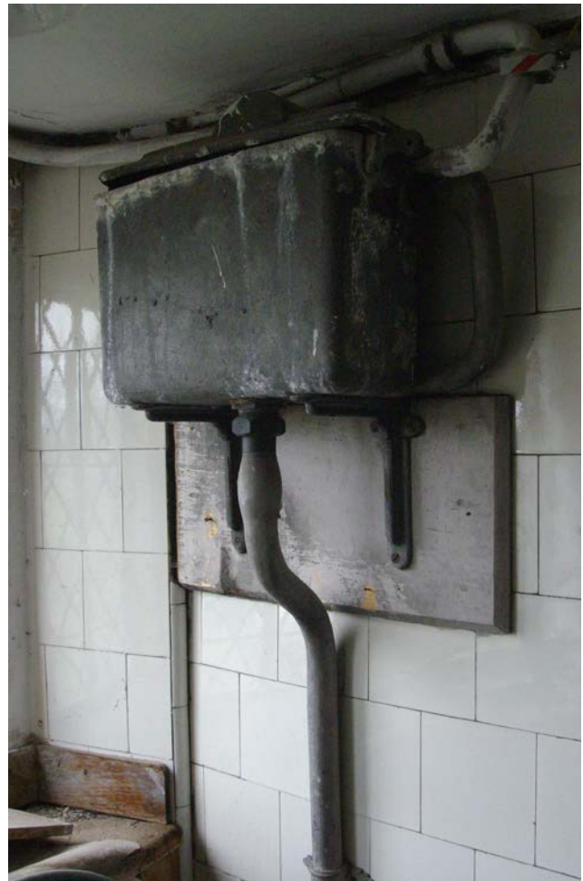
Figure 1: Lead water pipe for WC with wiped soldered joint below cistern. Photo: Douglas D Kent
